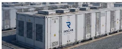
● GRID-SIDE STANDALONE BESS
